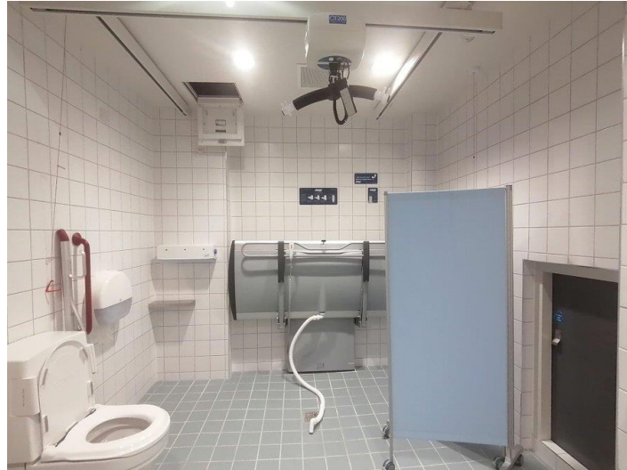
Figure 3a Changing Places Toilet Facility, UCC
